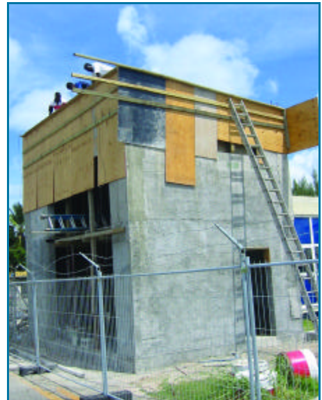
Workmen dotting I's on the roof of the new wind station, which should be completed by November.
